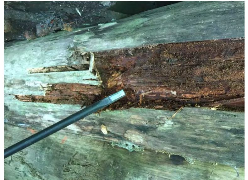
Top face log condition on right abutment
