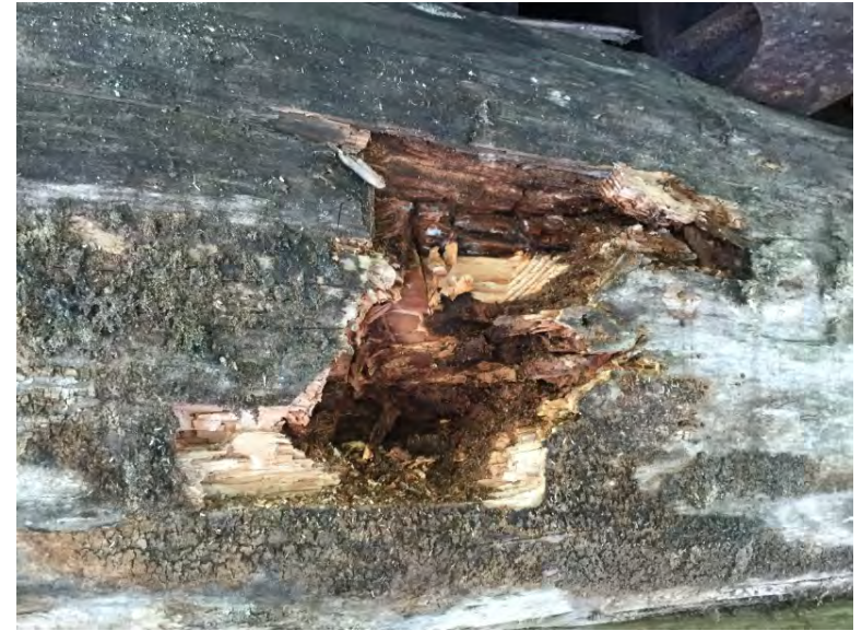
Top face log condition on left abutment 70mm rot at upstream girder bearing location
