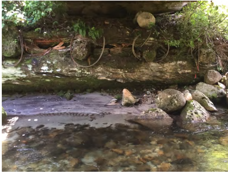
Old crib condition on right abutment condition is poor
